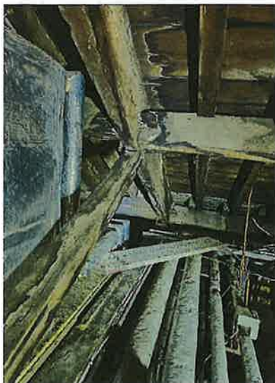
Previous Water Penetration
